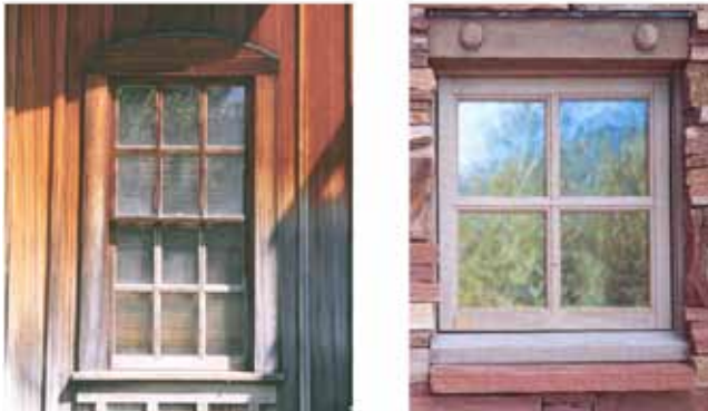
Windows set within wood walls are to be trimmed on all sides, with divided lines.
